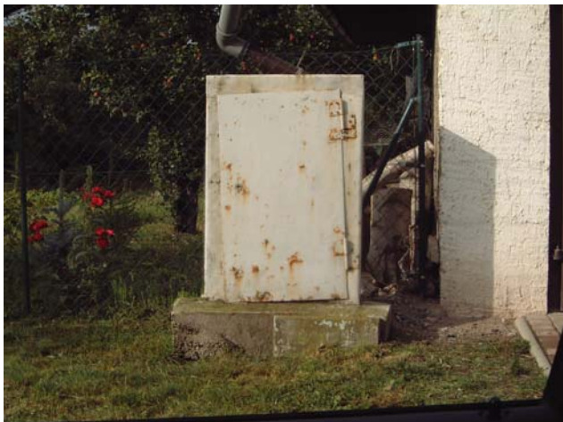
rusty cable distribution cabinet made of metal sheets (not SMC)
